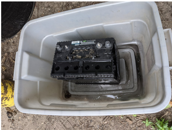
Photo 1: Ruptured Exide battery
